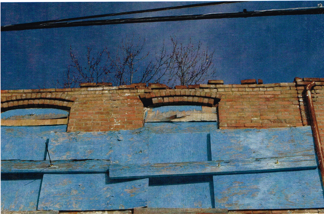
Photo 3 showing missing brick in upper floor window arch.
