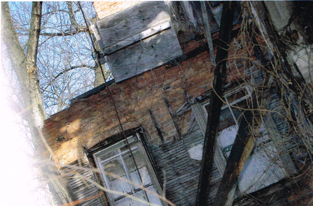
Photo 5 showing the collapsed interior of 104 Washington Street. The wall in the center of the photo is the back wall of the building behind 104 Washington Street, viewable, as the rear wall of 104 Washington Street has partially collapsed.
