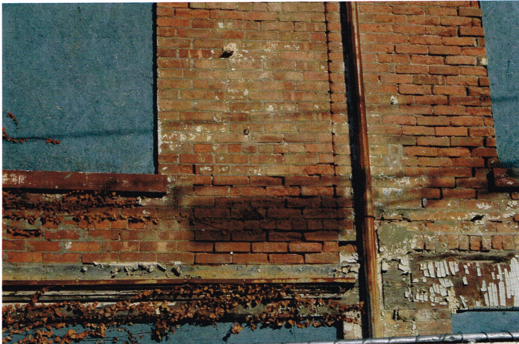
Photo 4 showing degraded state of brick work in walls.
